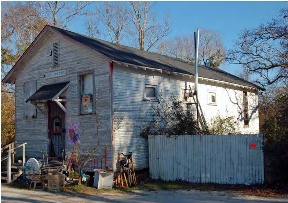
Plate 44. Scotts Hill Rosenwald School, Front (West) and Side (South) Elevations, Looking Northeast.
