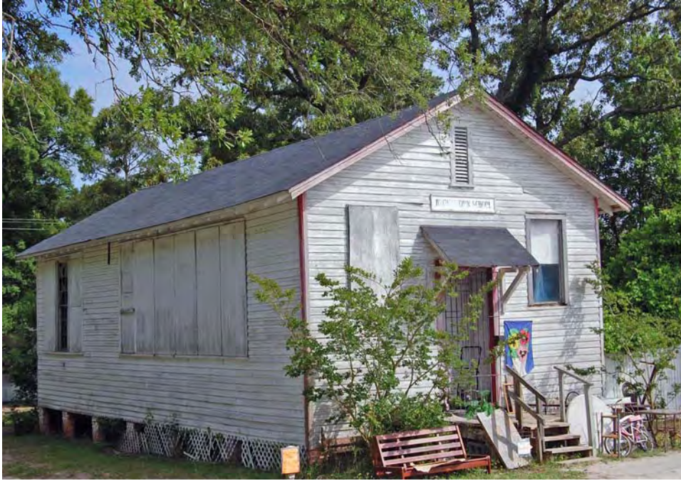
Plate 43. Scotts Hill Rosenwald School, Front (West) and Side (North) Elevations, Looking Southeast.
